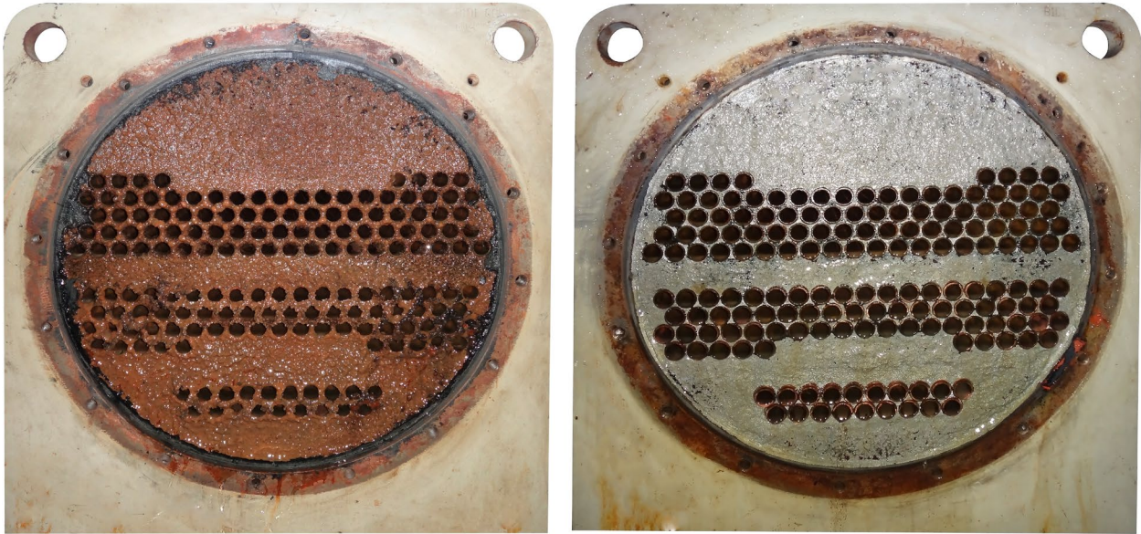
Figure 2: Heat exchanger with fouling, and after cleaning
